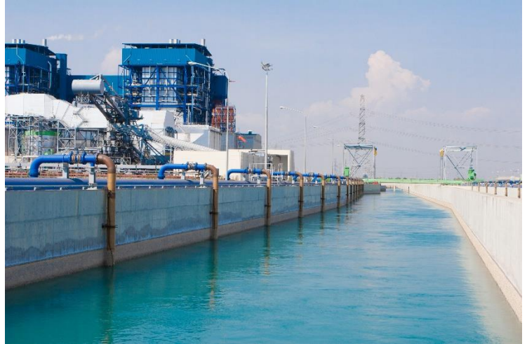
Figure 1 - Wastewater treatment at a petrochemical site
